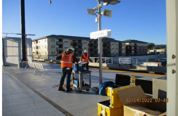
Photo 2 - OCS Grounding Testing.
