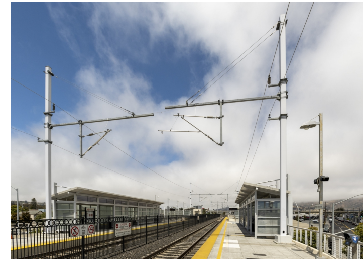
Overhead Catenary System
