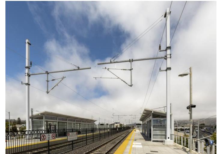
Overhead Catenary System
