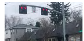
Pedestrian Hybrid Beacon for bicyclists and pedestrians to cross Newbridge St at Saratoga Ave
