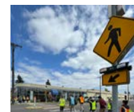
Rectangular Rapid Flashing Beacons (RRFBs)
